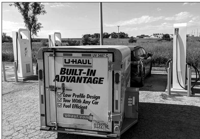
The Electrify America array at the Casey’s store in Williamsburg, Iowa, provided easy-in access.
